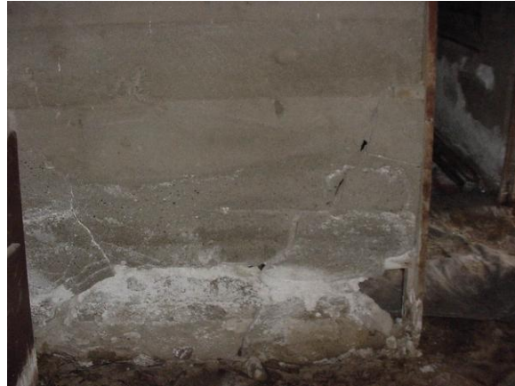
Above: Alkali damaged concrete wall. Left: Interior stem wall at passage.
