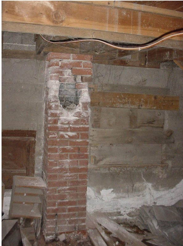
Left: Chimney at basement, deteriorated by alkali and exposure to air.
