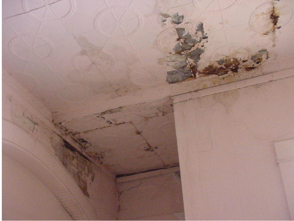
Significant paint peeling, rust, and deterioration of tin panels at south end of former chancel
