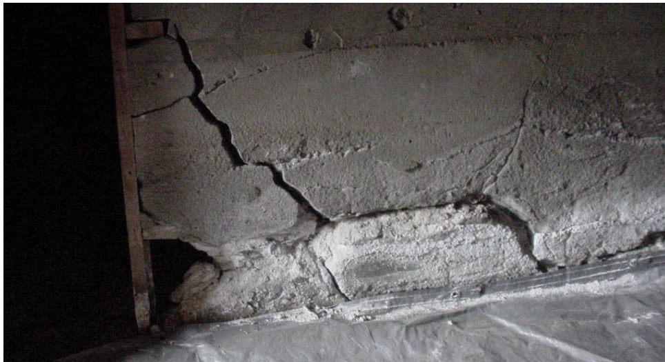
Above: Southeast corner of stem wall, with large cracks and crumbling.
