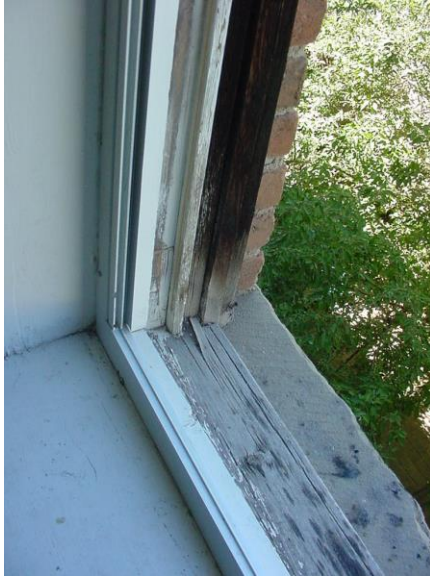
Upper level window: rotted sill.
