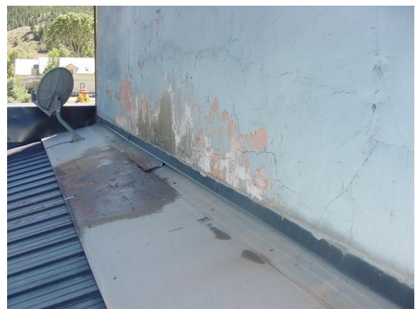
Sheet metal flashing.
