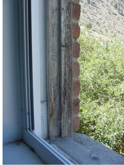
Upper level window: rotted trim.
