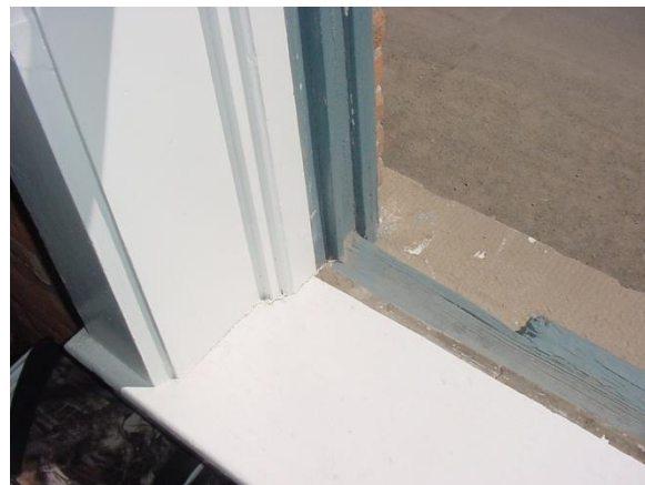
Upper level window: damaged wood trim.
