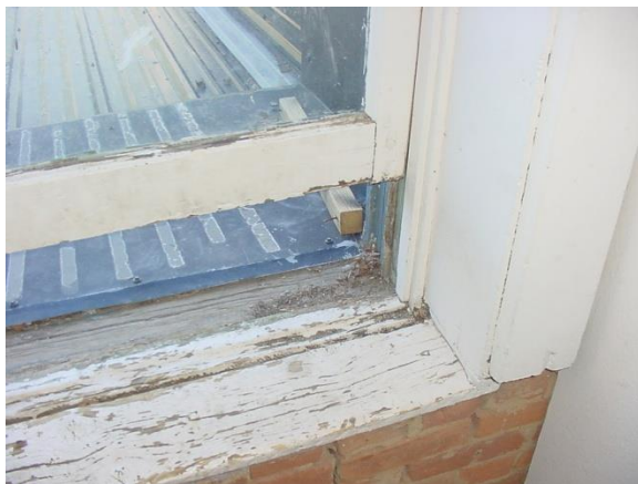
Upper level window: rotted sill
