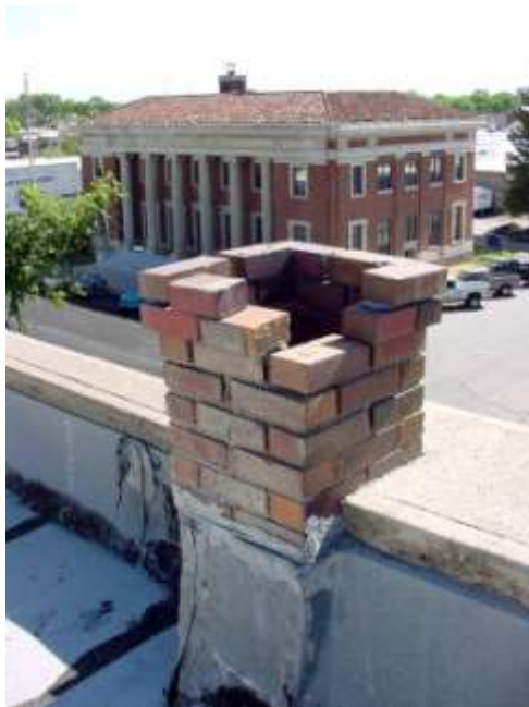
Chimney at east battlement. Note potentially perilous placement of bricks.
