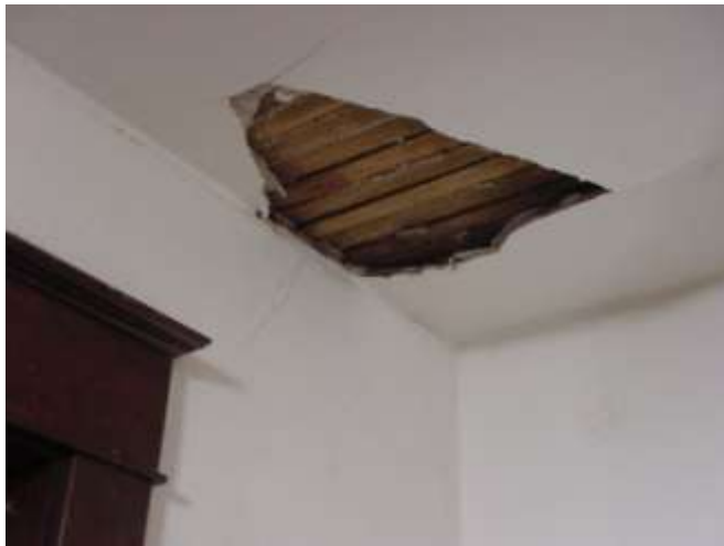
Above: Failed plaster in upper level. Right: Plaster bracket at the ceiling of the sanctuary.
