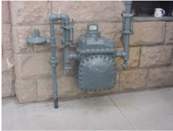
Gas meter at west elevation.
