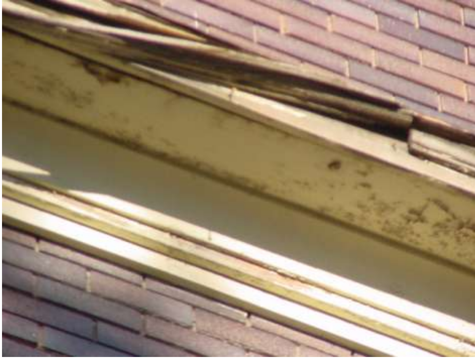
Extensive dry rot at wood cornices.
