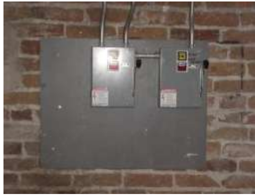
Electrical subpanels in boiler room.
