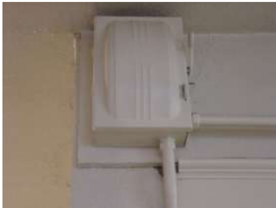
Electrical shutoff in kitchen.
