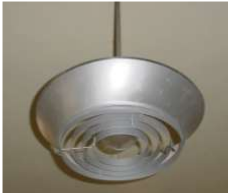
Light fixture in hall.
