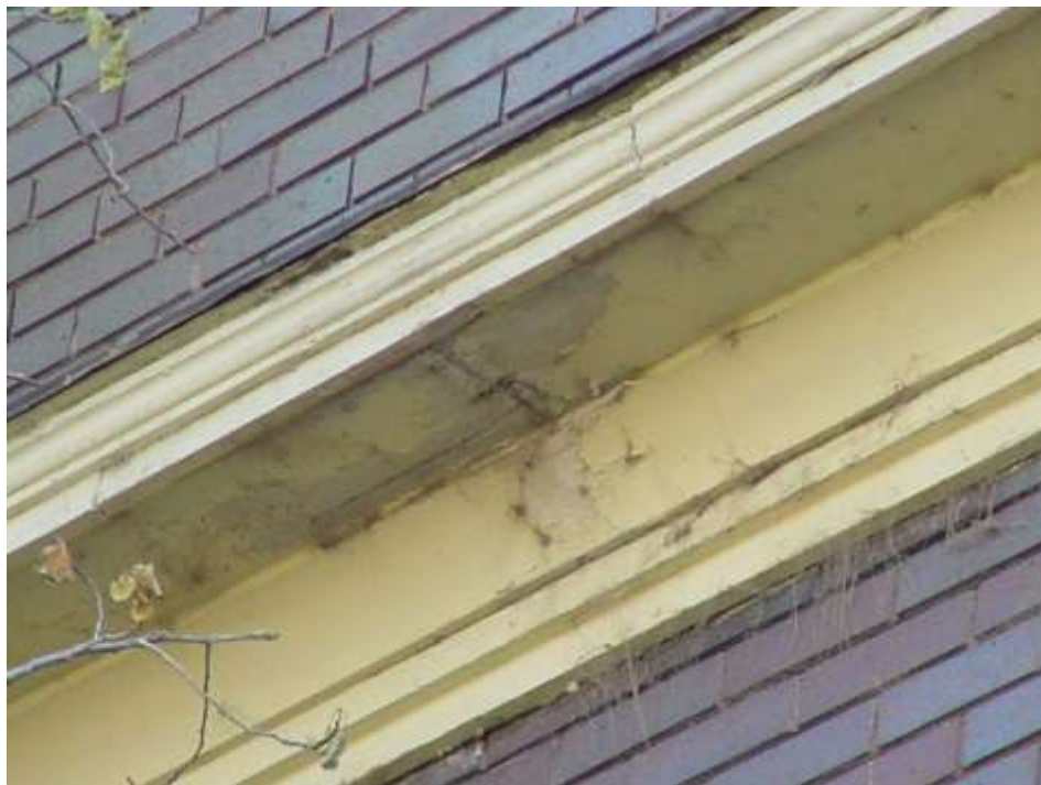
Below: Extensive dry rot at wood cornices.
