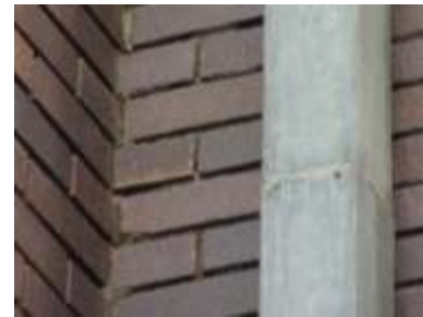
Leader at west side of south elevation. Note loss of mortar at brick.
