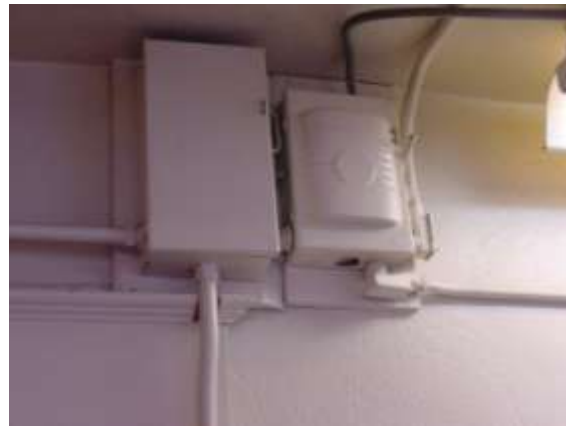
Electrical subpanel and shutoff in kitchen.
