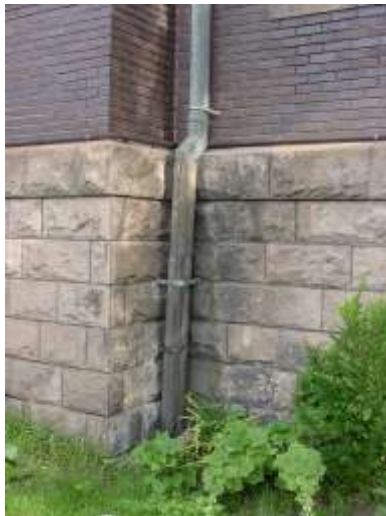
Leader at west side of south elevation. Note the dark, discolored rhyolite stone.
