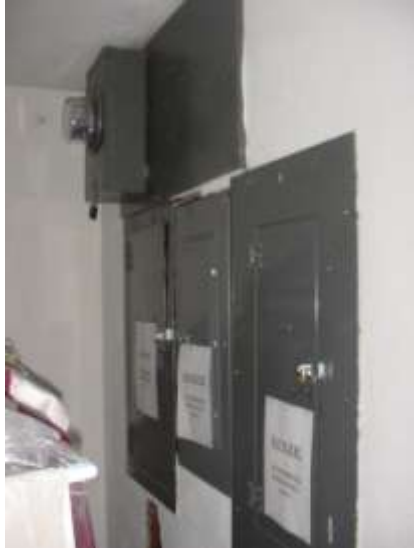
Electrical meter and panels.
