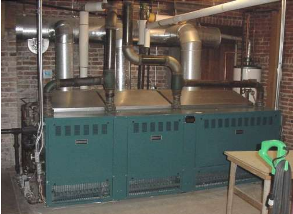
Burnham boiler. Note hot water tank at right.
