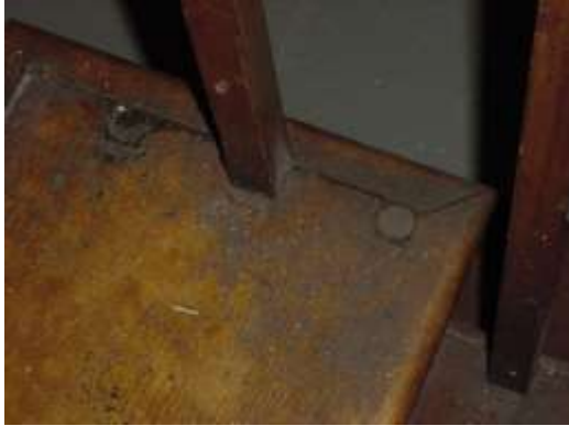
Stair with split tread at lower level.
