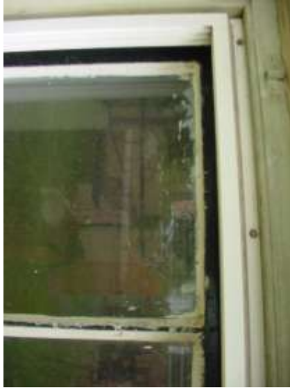
Left: Window at north elevation basement level. Note poor application of glazing putty on window.
