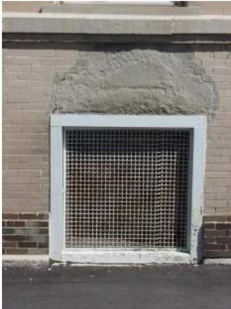
Left: Condition of area above vent grille on west face of building. This area must have all cement removed and replaced with brick to match its surroundings.
