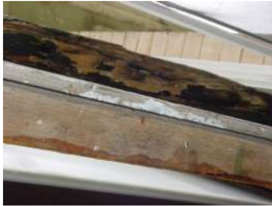
Rotted sash at stair landing window
