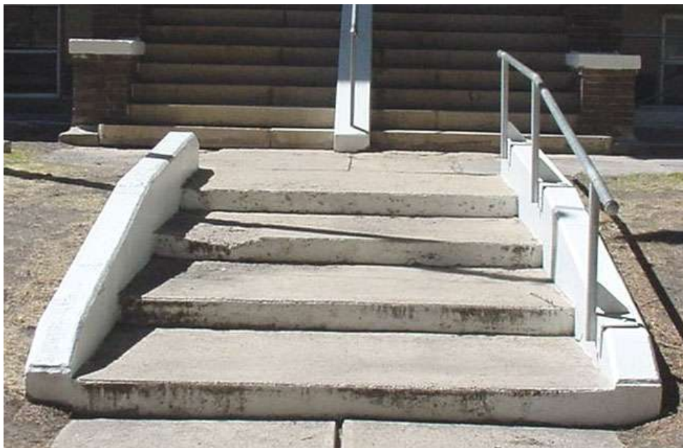
Front (east) site stair. Date constructed unknown. Note crumbling on third tread and non-original pipe rail.
