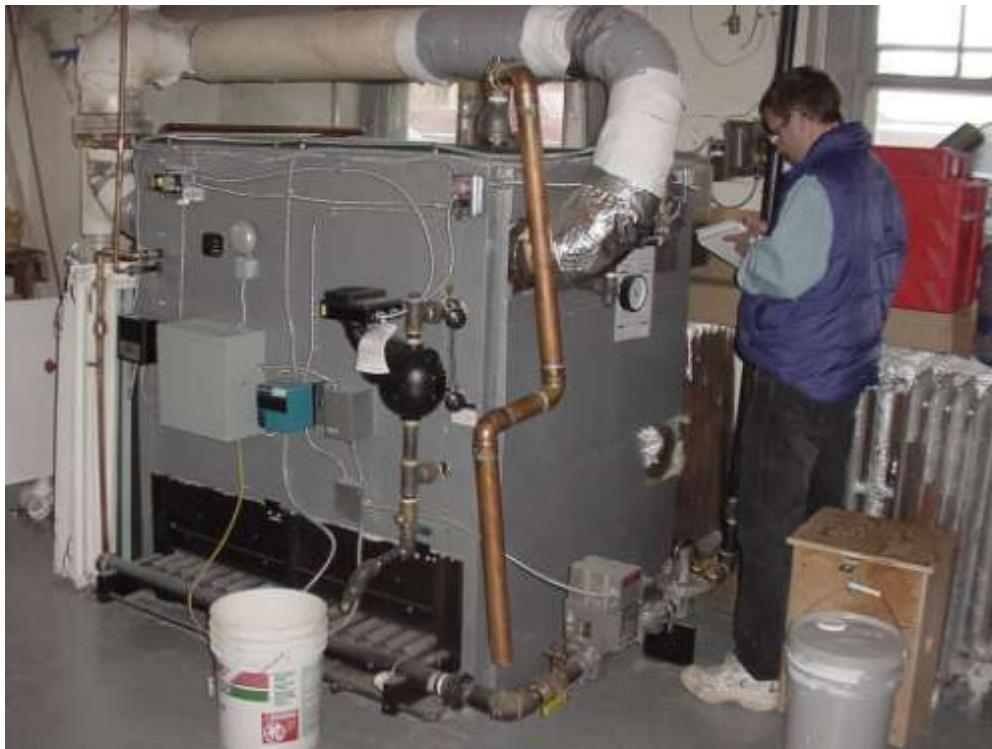
Peerless cast iron boiler, 2001
