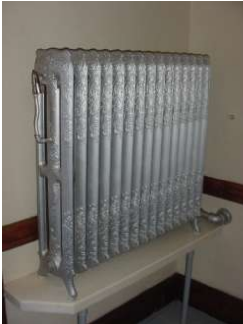
Left: Cast iron radiator, typical throughout building.
