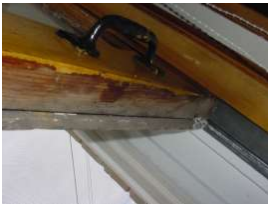
Rotted sash at second floor window
