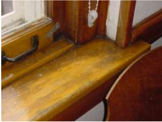
Rotted window sill at second floor
