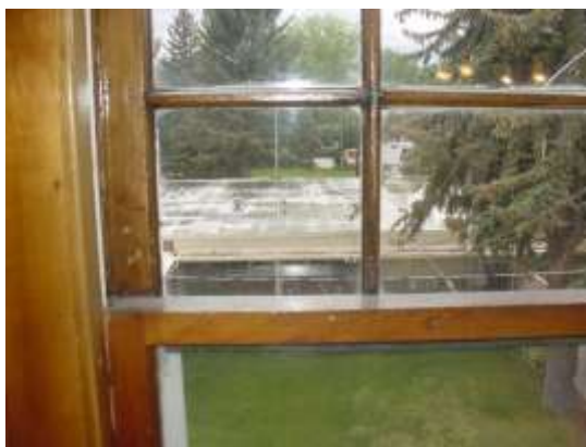
Cracked panes and bowing rails at second floor window
