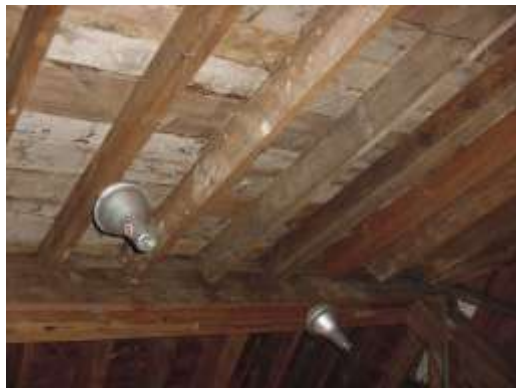
2x8 wood rafters and 2x12 decking, with cement-covered faces. Note primitive fire suppression units.
