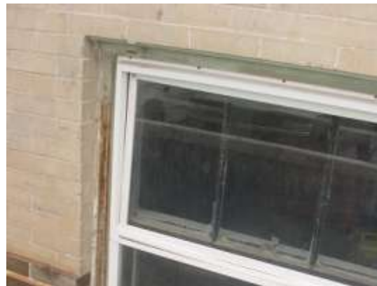
Rotted exterior trim at basement window
