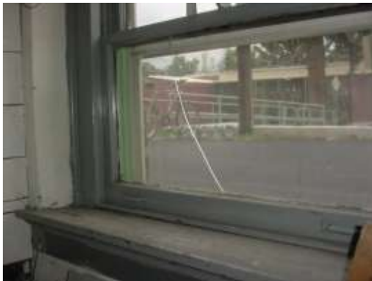
Cracked window at basement level
