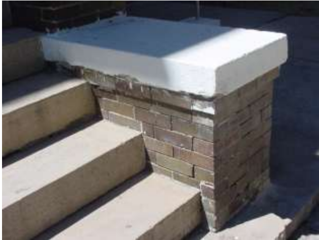
Purple brick at stoop. Note improper painting of abutment.
